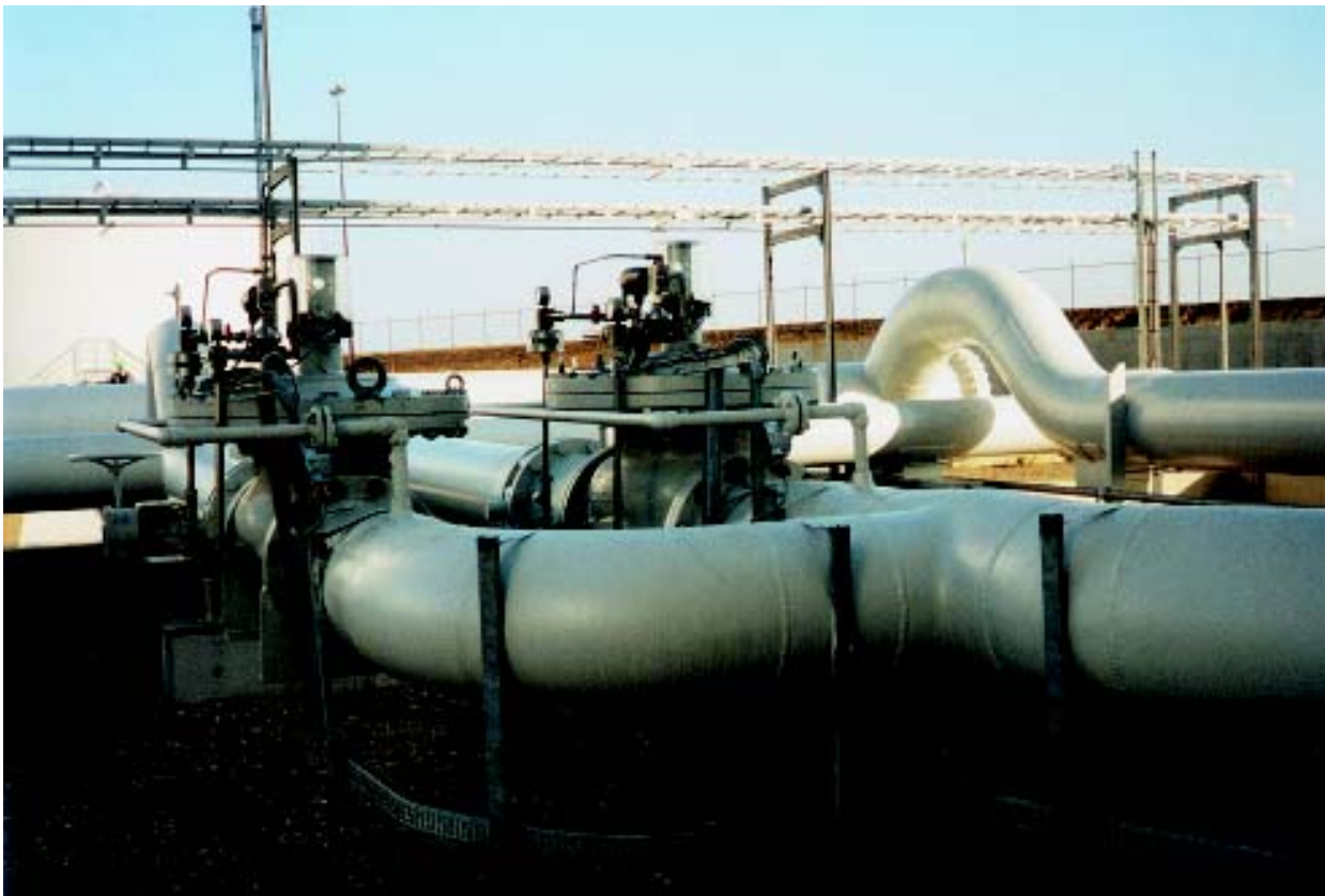
Multi-Purpose Control Valve Type HV (in a Kerosene Pipeline DN 350 of an international airport)
