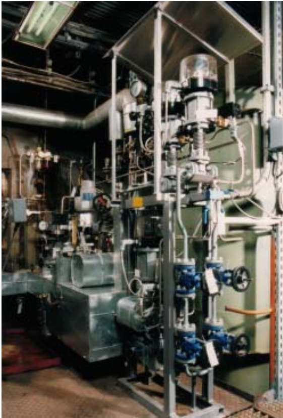
Heating Oil Burner Station for a large-scale, lignite-fired power plant
